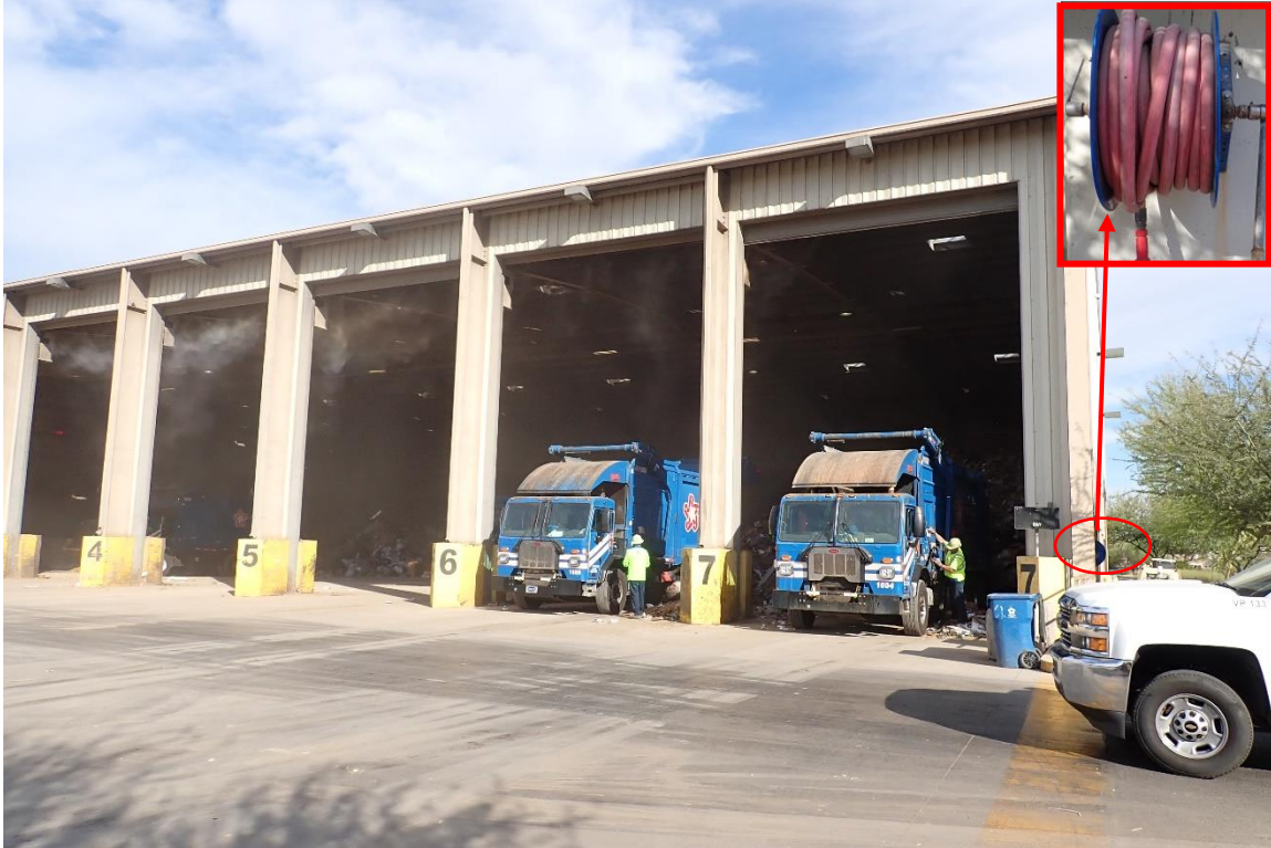
Cave Creek site with five of the seven bays, misting system on-1" fire hose circled in red
